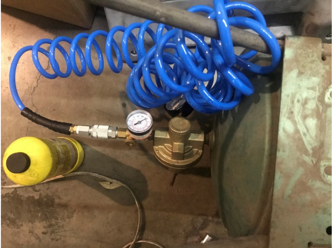
Figure 8.4-3 ¼" Compressed Air Hose on Water Tank
